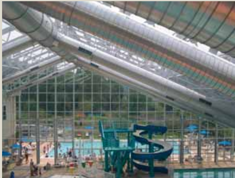
Maryland manufacturer Wm. H. Brady supplied six additional dual-wall spiral-duct systems located throughout the athletic center. The duct has 1-inch insulation and was manufactured from galvanealed material so it could be painted to match the interior décor.
